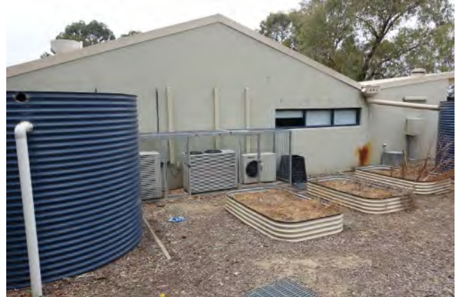
Figure 22. Tanks and dried out edible gardens Tamara Children's Centre, Cranebrook. Photo: Helen Armstrong December 2015
