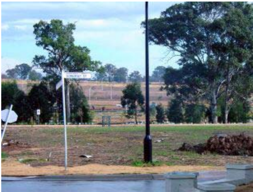
The next stage: streets have been laid out, including the street lights, but the houses are still to be built
