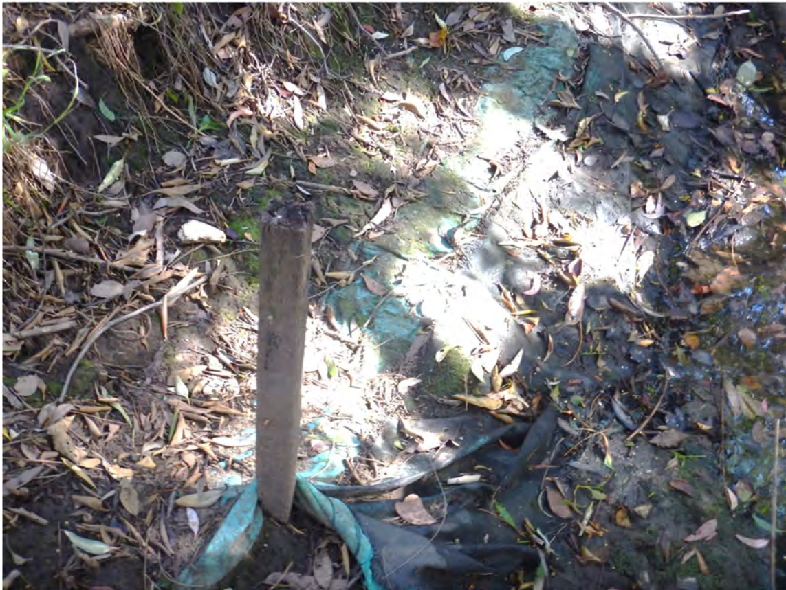
Plate 5. Compromised sediment retention fencing along Vineyard Creek
