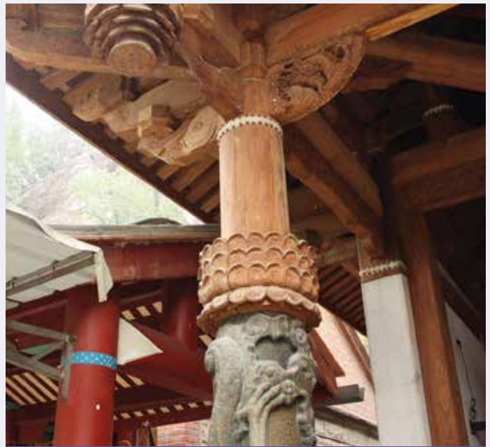
Temple at Xiamen, China, where the wooden roof structure has been replaced but the old stone pillar remains intact
