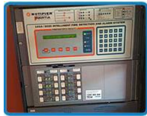
Fire Panel Isolation
